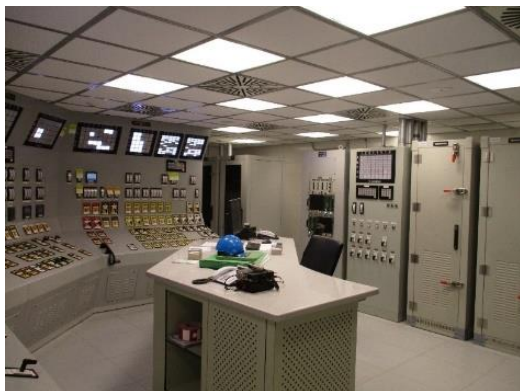
Emergency Control Room
